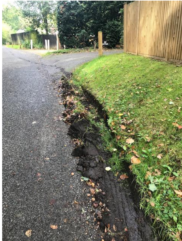
Damage done to private verge
