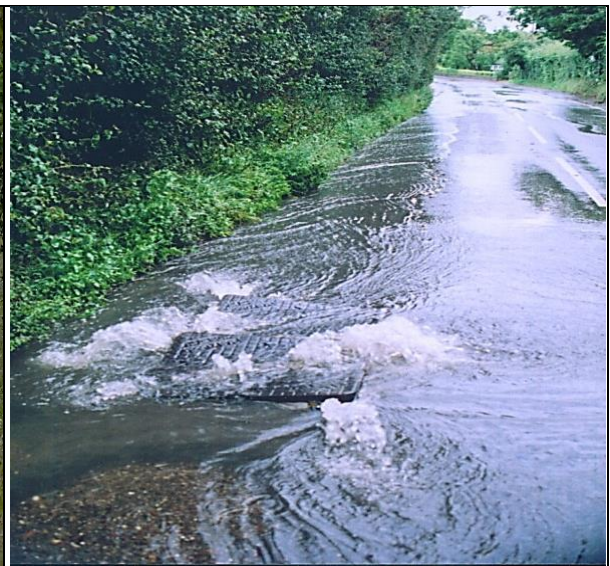
Figure 2 Manholes near The Hautboy, Ockham
